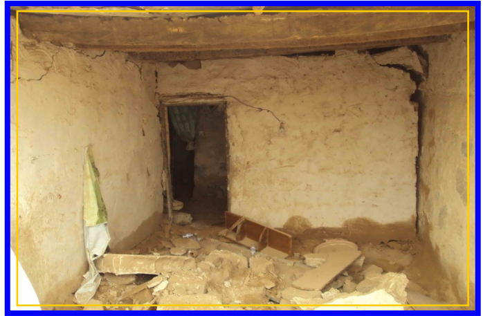
Flood-Damaged Home in Kerbala
